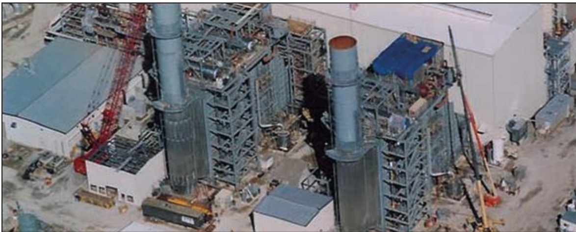
Duke Energy Plant
